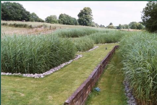
Reed Bed Waste Water Treatment
